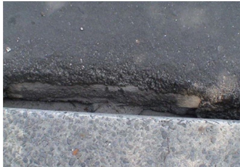
Roadway Surfacing creating a Potential Hazard for cyclists near curb
